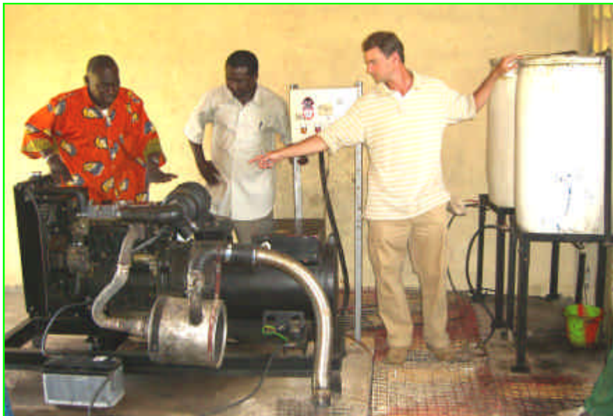
John visits an electric generator that runs on locally-grown jatropha biodiesel.
